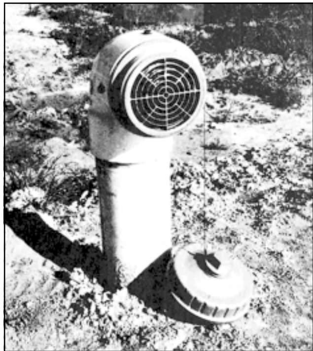
WATER PRESSURE: A Dry Fire Hydrant*
